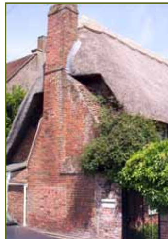
Figure 31 Tumbled brickwork on a gable end stack
